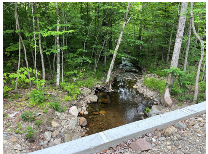
And looking downstream from the new Stream Smart crossing. Notice how the new streambanks connect to the existing streambanks outside of the crossing.
