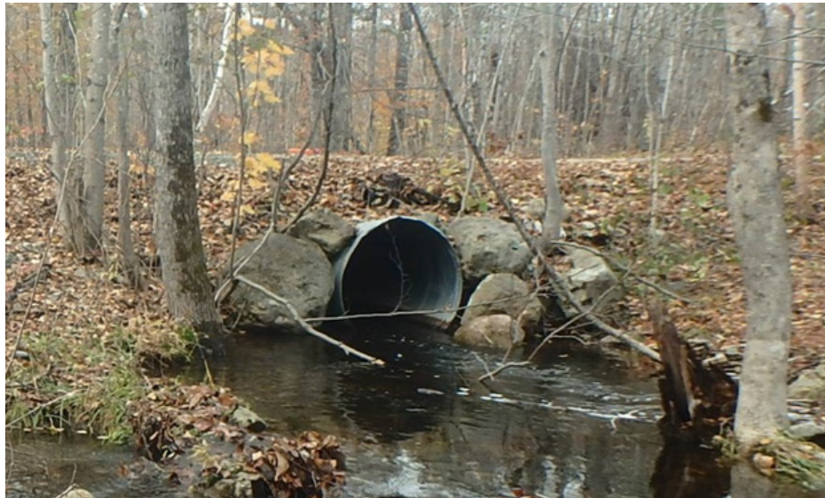
Another undersized crossing
